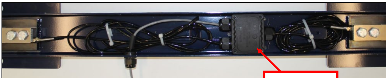
Internal Junction Box
